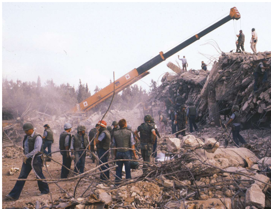
Below: Marines and sailors assist as heavy equipment is brought in to help in rescue and recovery operations after the Beirut terrorist bombing, late October 1983.
